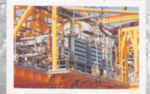
Kirloskar Balanced Opposed, Oil free, Air Compressor Package on offshore drilling platform at ONGC.
