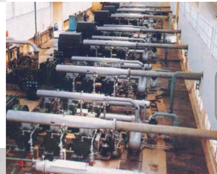
7 Nos. Balanced Opposed Piston Air Compressors of 99.60 M 3 /min capacity each, installed at NALCO Angul.
